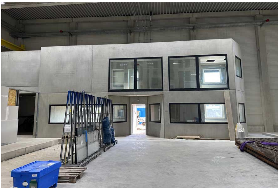
Caption: The new Menzel Elektromotoren plant is rapidly progressing towards its on-schedule completion (pictured: test field cabin with customer lounge)
